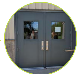
Hollow Metal Door with Hollow Metal Frame
